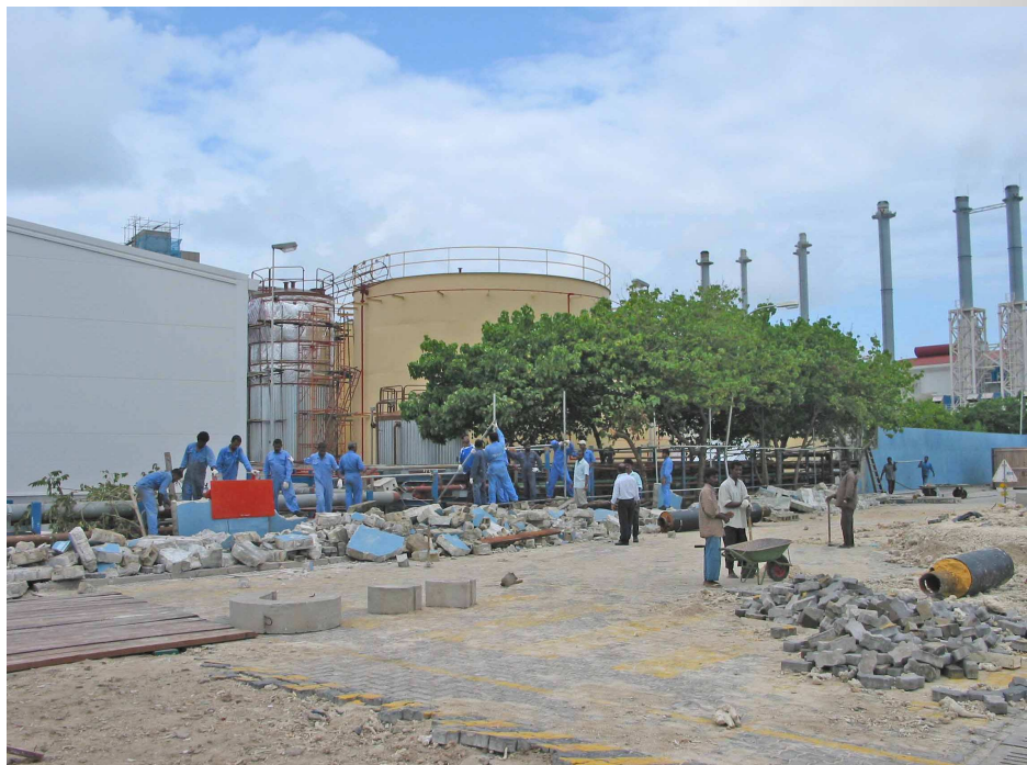
Effects of Tsunami (26. Dec. 2004) on HFO Conversion works Fuel pipe rack, Fuel Treatment House, HFO service & storage tank
